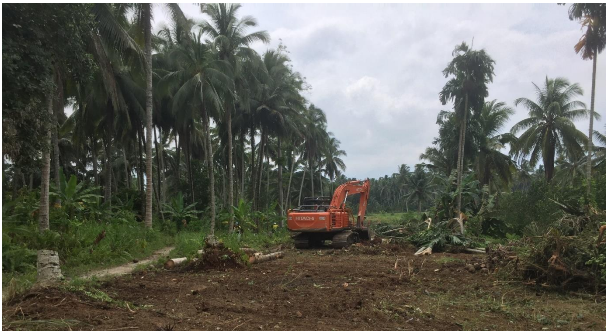
Figure 15: Clearing and grubbing activities for the upgrades to the Government Access Road
